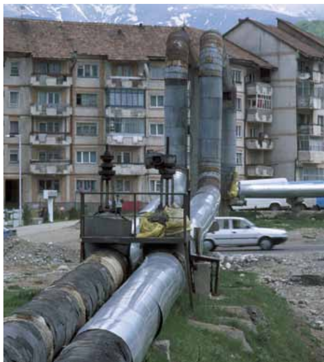
Town heating pipes, Romania
